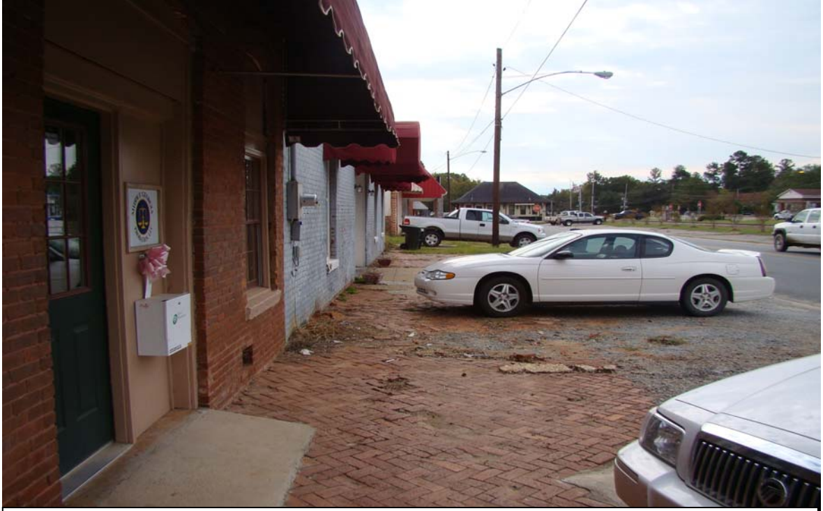
Photo 7: Deteriorating sidewalk due to vehicles parking on surface.
